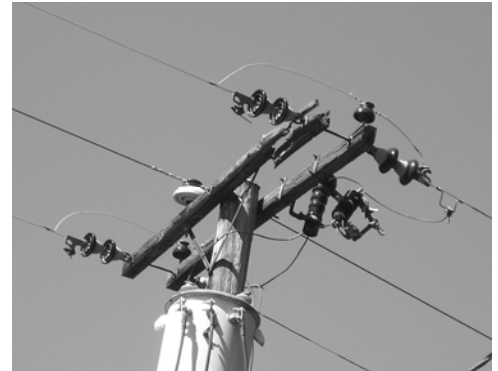
SUPPORT ARM ON POLE WITH A POWER LINE THAT IS SPLIT AND FALLING APART.
