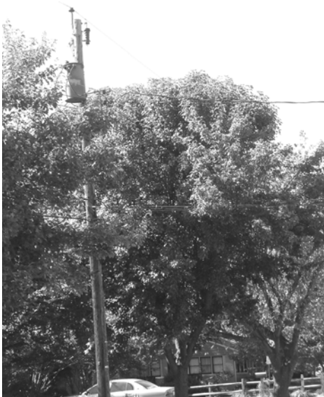
TREE GROWING AROUND LINES
